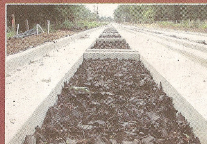
The voids between concrete spacers running along the centre of the busway were filled in using shredded tyres as agreed by the council.
