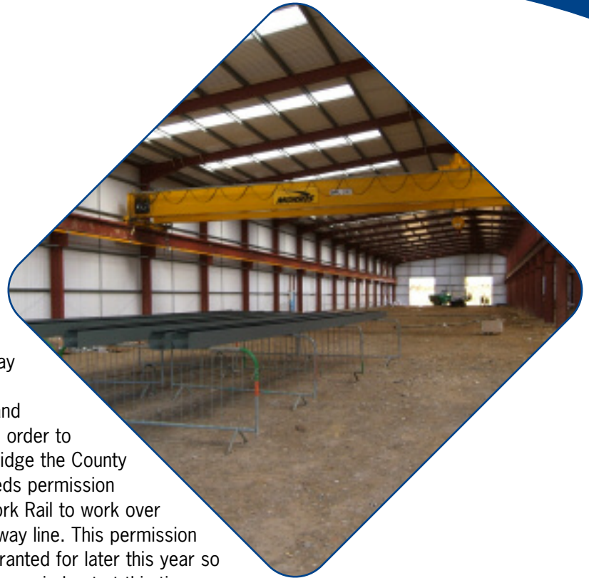
Work is still underway to complete the large shed where the guideway beams will be made.
